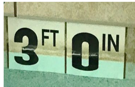
Waterline Tile in Need of Cleaning
