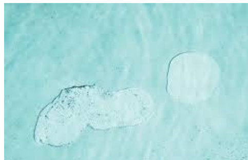
Deteriorated Pool Plaster Caused by Etching
